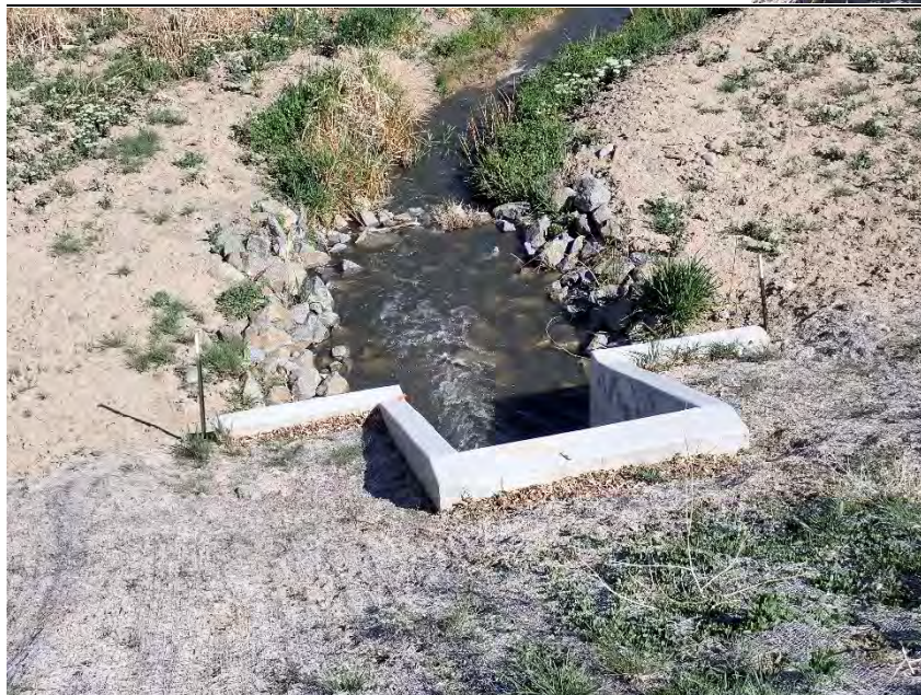
Outlet flowing during gate exercise. Note discolored water.
